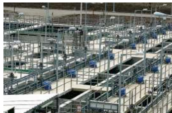
The Eskol Water Filtration Plant, Northern Israel ©The Times of Israel
